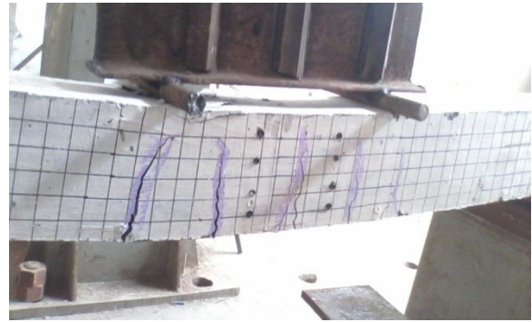
a) Crack pattern for control mix M1
